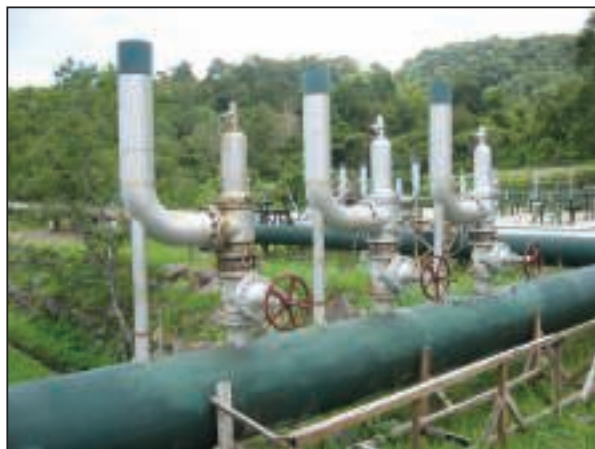
FIGURE 2. Installation of rupture discs upstream of relief valves allows for in-situ calibration testing of relief valves
