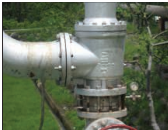
FIGURE 3. Rupture discs can prevent leakage through the relief valve and prevent corrosion of relief-valve internals when positioned on the process side of a valve
